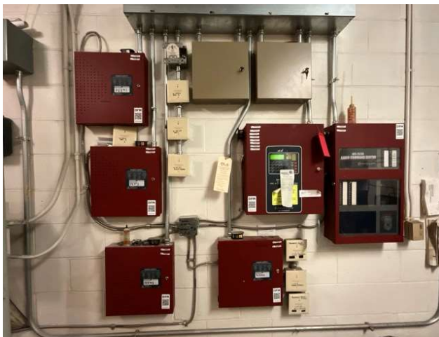
29 - FIRE ALARM PANEL
