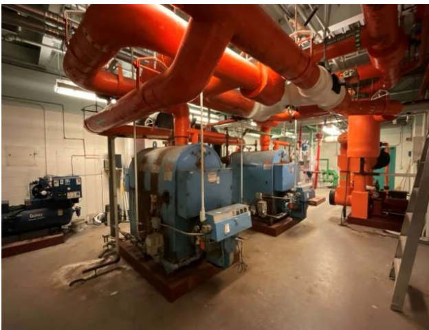
23 - MAIN MECHANICAL ROOM
