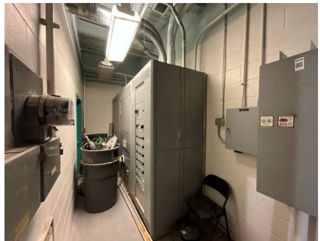
24 - MAIN ELECTRICAL ROOM
